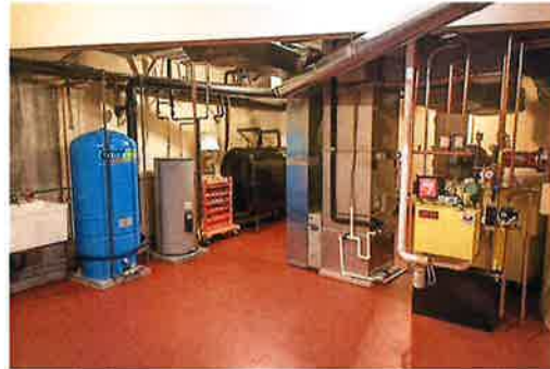
Systems Room in Octagon
