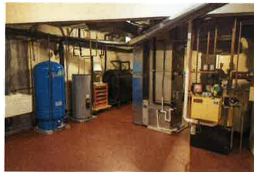
Systems Room in Octagon
