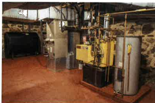
Systems Room in Main House
