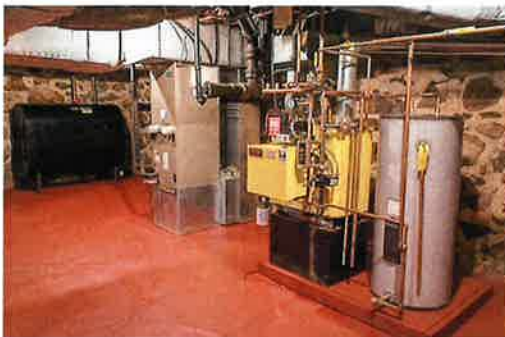
Systems Room in Main House
